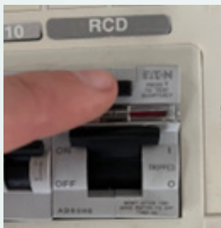
Pressing the test button on RCD
