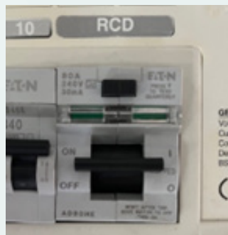
RCD with lever in the tripped position
