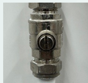
Isolation valve in open position
