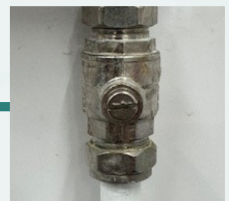
Isolation valve in closed position
